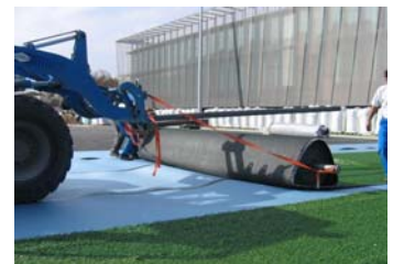
The artificial turf is rolled out after the foam sheets have been bonded together.
