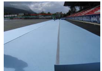
Alveo Sports Layer is laid on the subbase on the football pitch.
